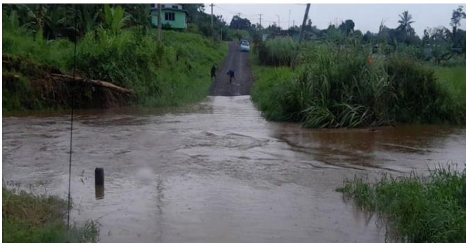
Figure E: Waisa Bridge on the 21 st . Source: National Disaster Management Office.
