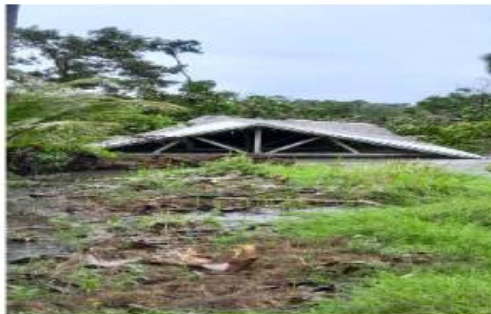
Dwelling house destroyed by the landslide at Kuratidalo Village, Small Ngella. Source: P-DOC CIP
