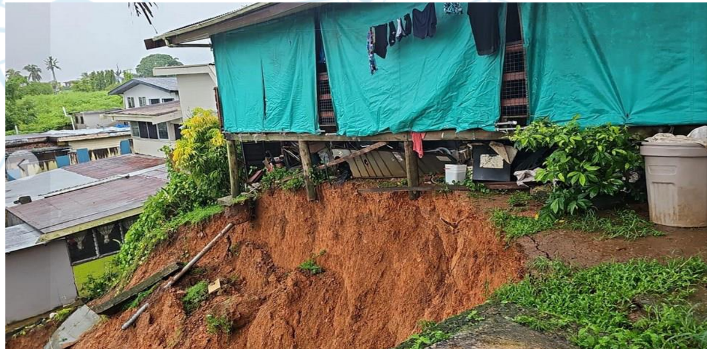
Landslide at Kula Street in Samabula, Central Division on 20th January, 2024. Source: National Disaster Management Office
