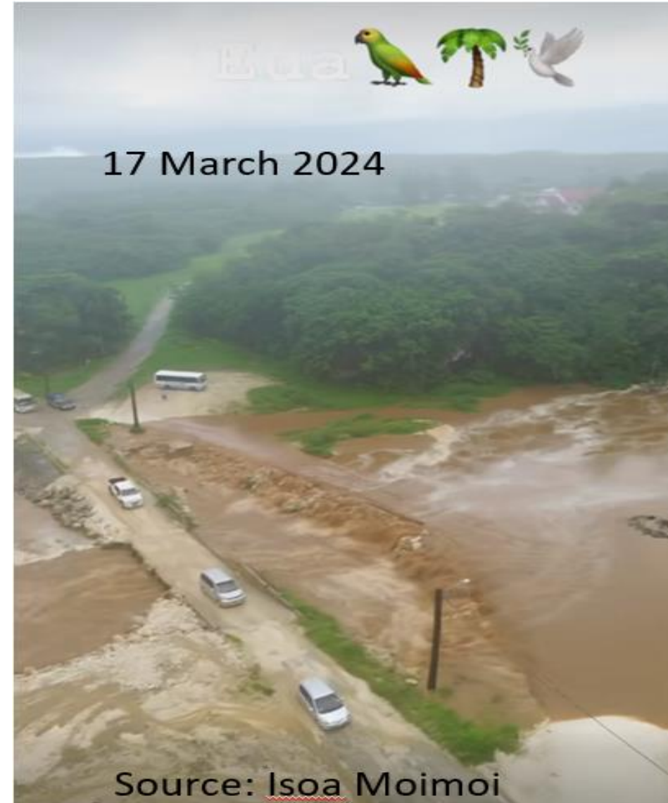
Fig 1. Damage to roads and bridge in 'Eua island due to heavy rain.
