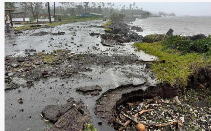
Coastal damage in Fiji from TC Yasa (source: Fiji Gov.)
