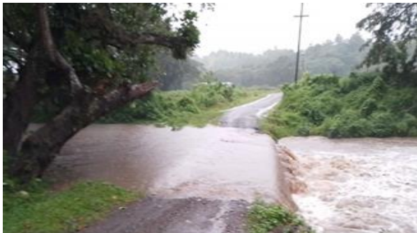
Lawai Crossing in Sigatoka inundated with floodwaters (Western Div.) - 30 th Dec 2022 (Source: Fiji Roads Authority)
