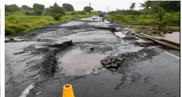
Rabulu road (Tavua) damaged due to continuous flooding (Western Div.) - 17 th Feb 2023 (Source: fijivillage)
