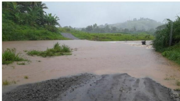
Marinitawa Crossing in Ba (Western Div.) – 30 th Dec 2022 (Source: Fiji Roads Authority)
