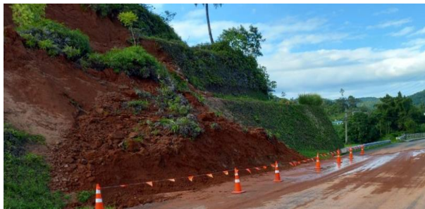
Landslide long Kings Road at Balekinaga Village, Rakiraki (Western Div.) - 11 th Mar 2023 (Source: Fiji Roads Authority)
