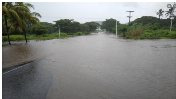
Flooded Natawa Bridge in Tavua (Western Div.) – 7 th Mar 2023 (Source: Fiji Roads Authority)
