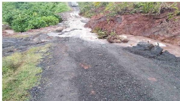
Landslide at Nakabuta settlement, Kubulau road, Wainunu, Bua (Northern Div.) - 21 st Feb 2023 (Source: The Fiji Times)
